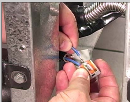
Figure 3: Connecting drain safety wiring.
